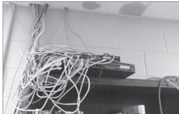
FIGURE 6–4 CABLING AT DALHART JUNIOR HIGH SCHOOL NOVEMBER 2016
